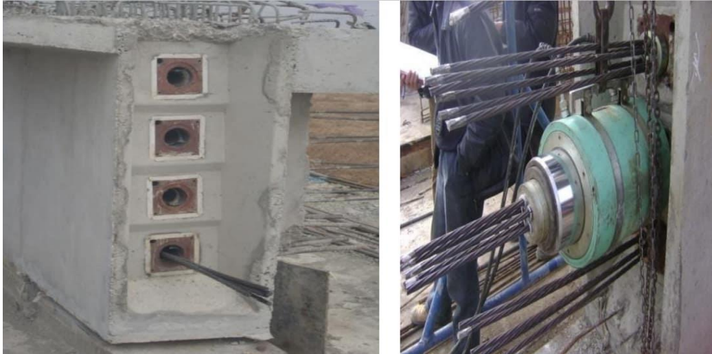
Figure 04. After the concrete has hardened, insertion of the cables into the ducts and their tensioning.
