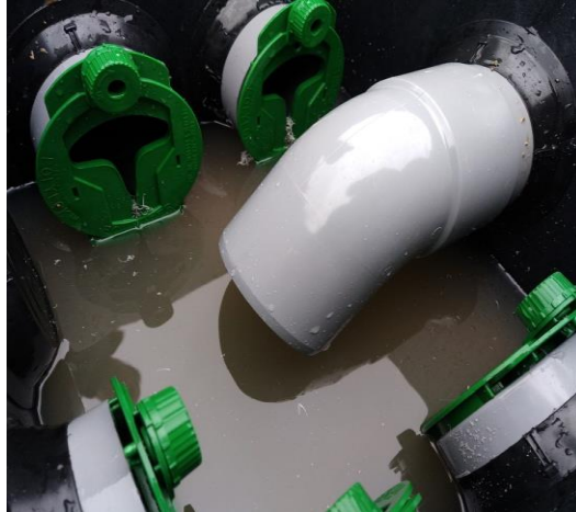
Figure 11 The inside view of DISTRIBUTION BOX
