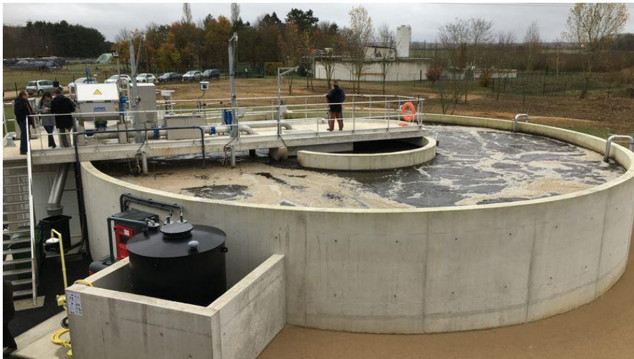
Figure 4 Activated sludge treatment plant
