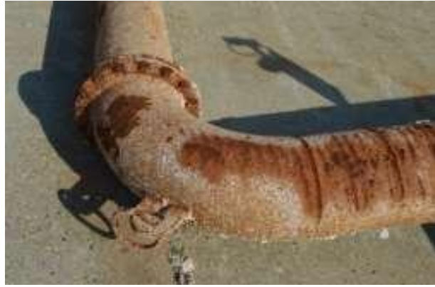
Figure I-19 : Figure.: La corrosion uniforme
