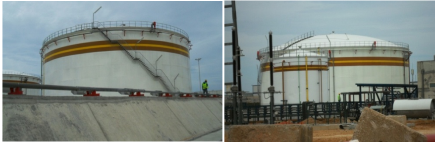
Fig.2.27 Bacs de stockage de gasoil.
