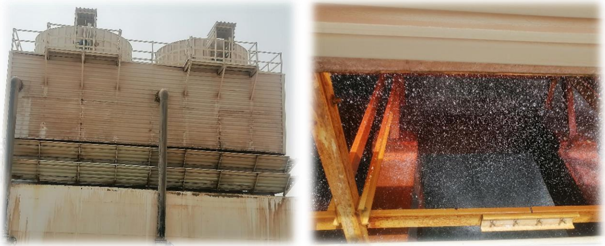
Figure III.2: Tour de refroidisse
