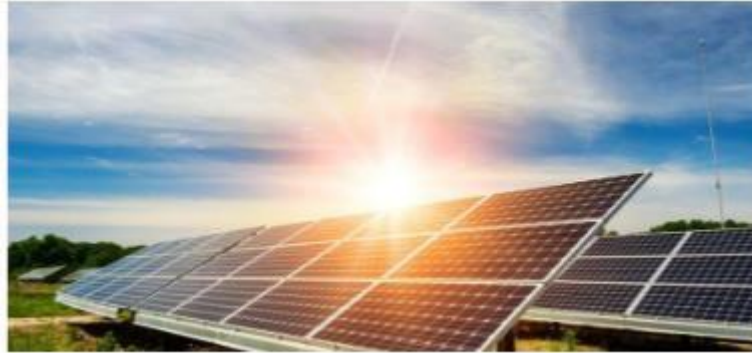
Figure (I.2) : Central solaire
