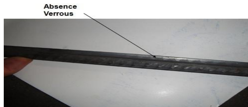
Figure IV.8 : Absence des verrous.
