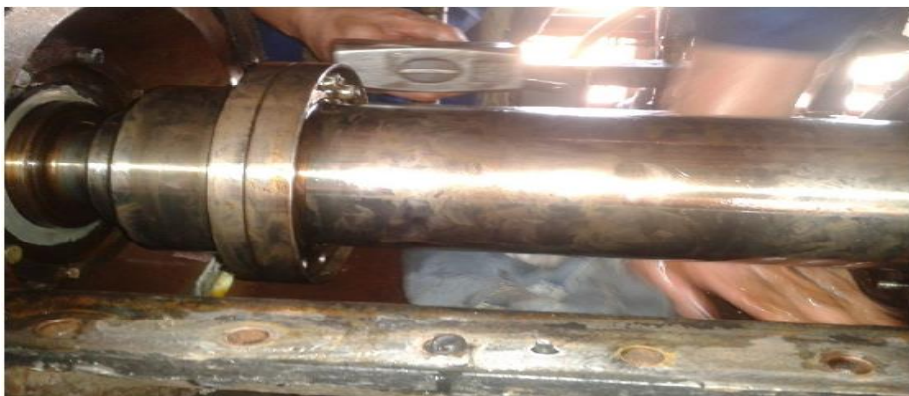
Figure IV.3: Moyeu et manchon cote turbine
