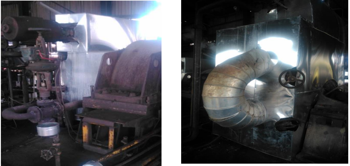
Figure III.5: Photos des turbines : (103-JBP ,103-JHP)
