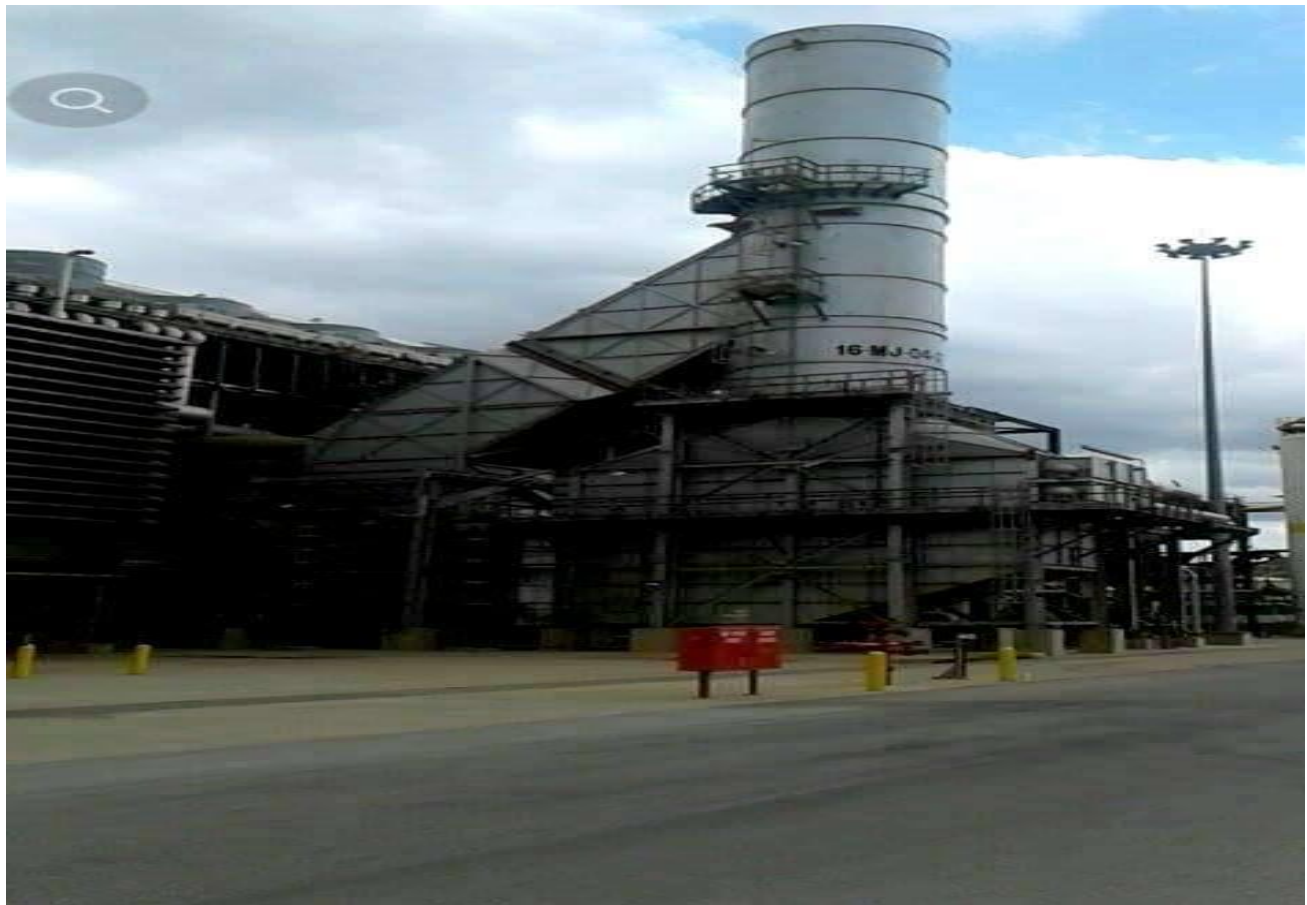
Figure II.5 turbine à gaz fram7 (MS7001EA) du complexe.
